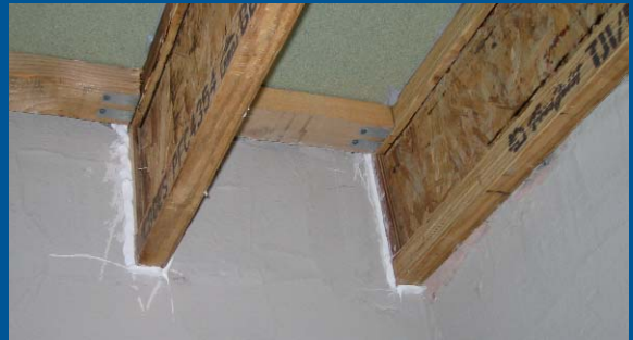
Built in joists with parging layer into the intermediate floor void, excess around the joists struck off and sealant applied (Stamford Brook development). Courtesy of Leeds Metropolitan University.
