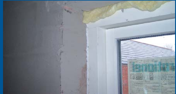
Window fitted and sealed to parging layer at the Stamford Brook development. Courtesy of Leeds Metropolitan University.
