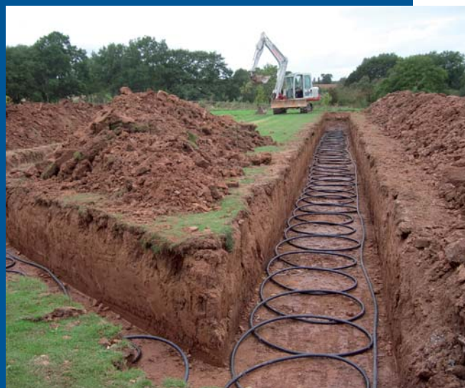
Ground source heat pumps are an effective way of reducing CO 2 emissions from heating and hot water. Courtesy of Kensa Heat Pumps.
